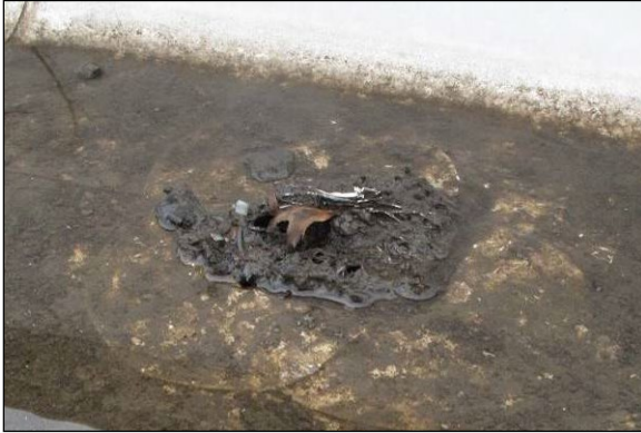
Figure 5. Organic growth and debris at a service facility roof drain
