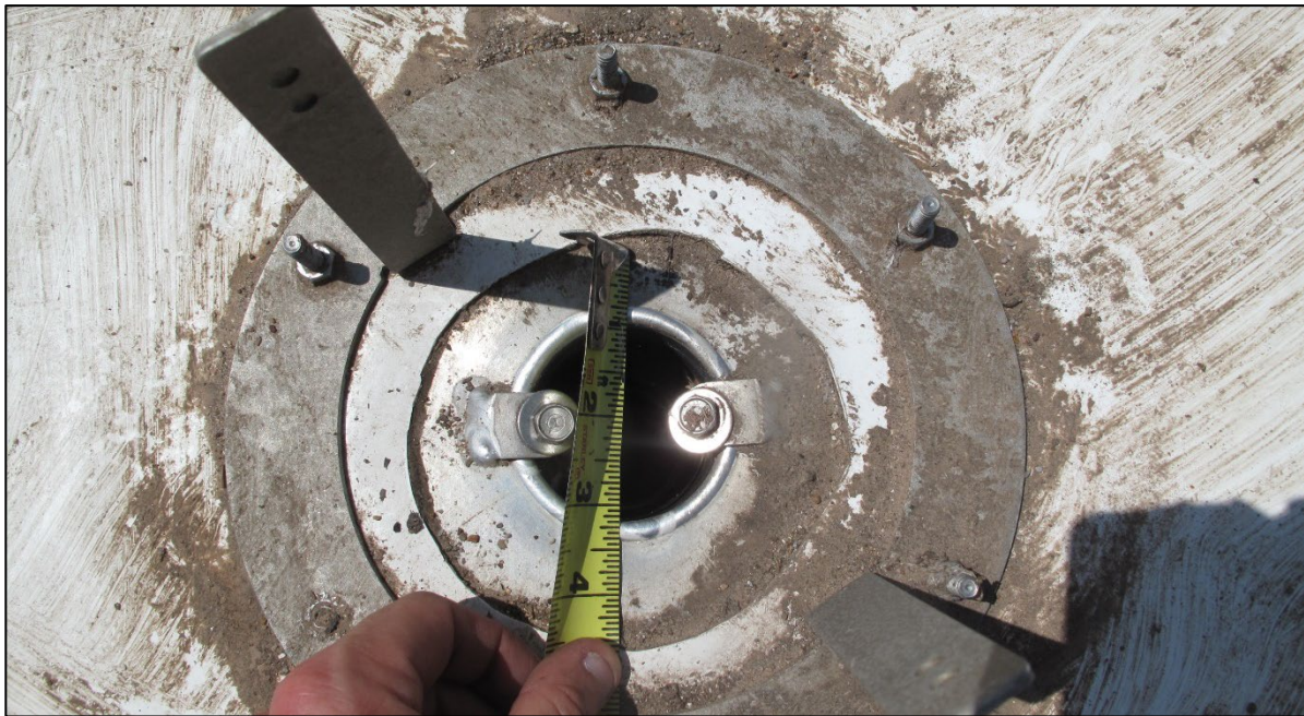
Figure 3. Modified drain inlet opening at the galleria
