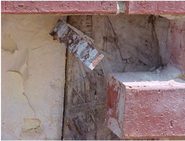
Figure 15. Veneer anchor corrosion at a structure less than one-year of age.
