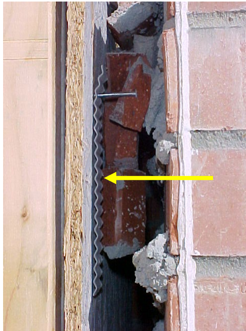
Figure 10: Veneer anchor that was detected during a survey but not anchored into the veneer.
