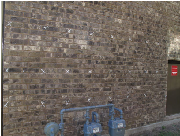
Figure 8: Overview of typical survey area at brick masonry veneer (anchors denoted with chalk "x" markings).
