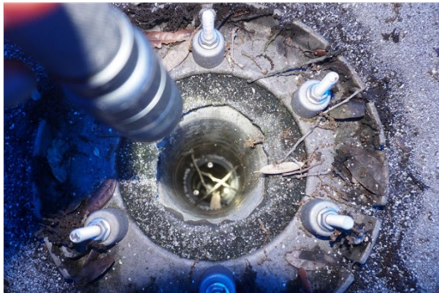
Figure 9. Debris and standing water at the drain pipe of the interior roof drain adjacent to the collapse area.
