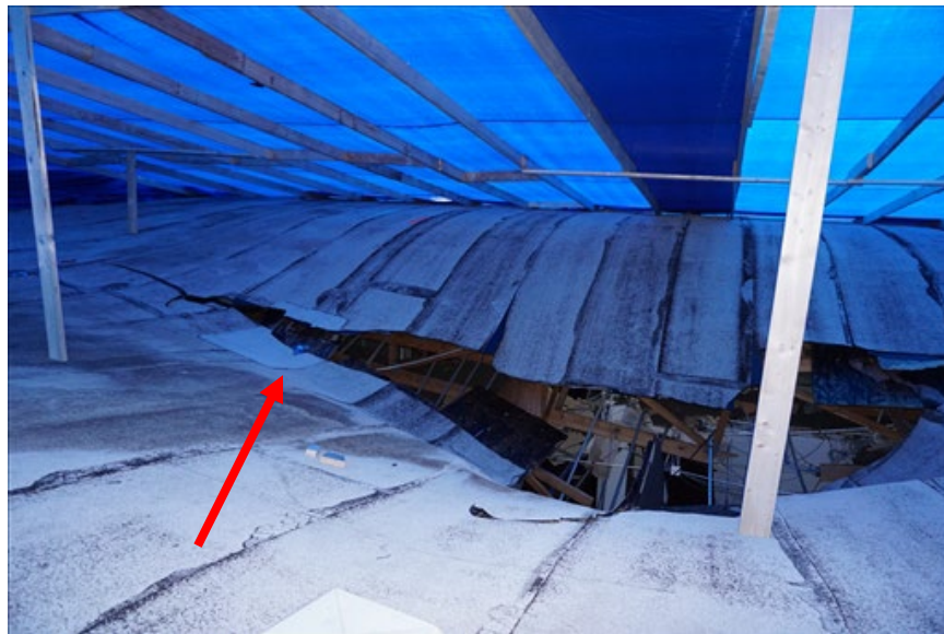
Figure 7. Collapse area at the roof. The blue tarp installed over this area is a temporary roof cover. The arrow indicates the approximate location of a previously abandoned drain.
