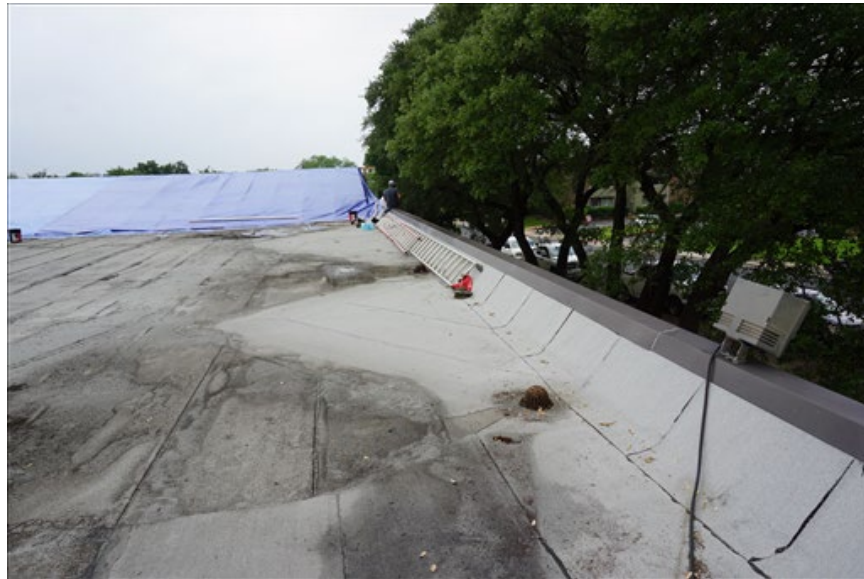
Figure 8. Perimeter roof drains. Note the lack of a secondary drainage system.
