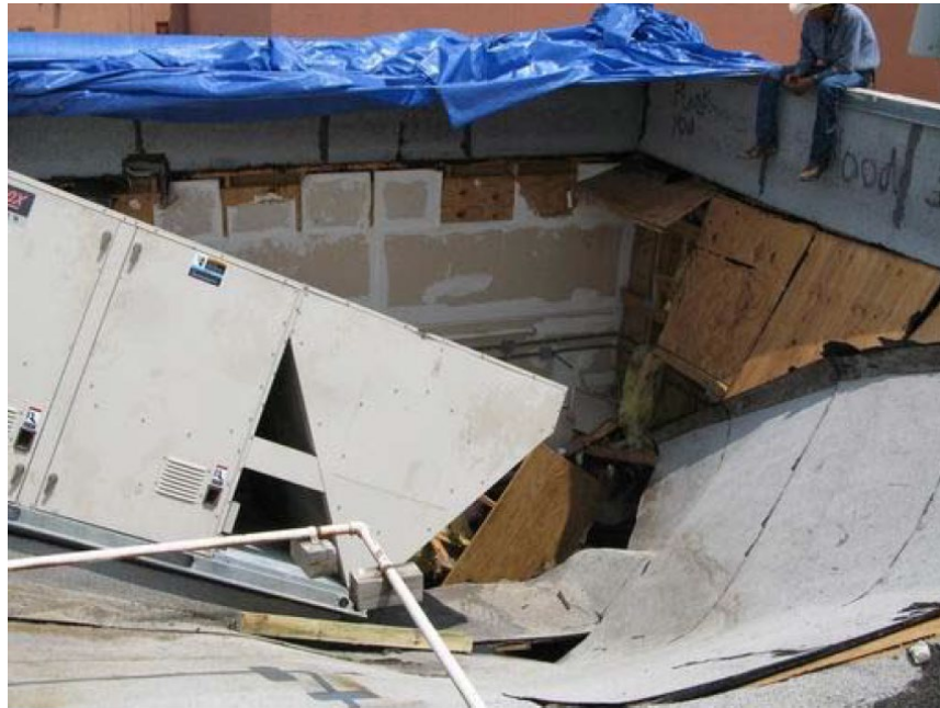
Figure 5. Collapsed roof framing at the building corner above the kitchen.
