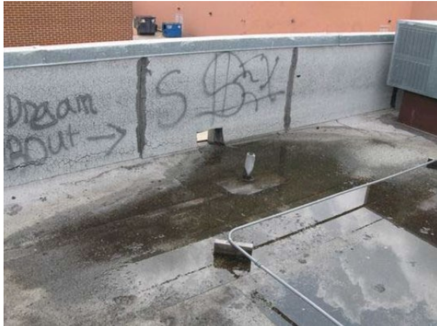
Figure 6. Standing water near the low side of the roof. Note the primary scupper drains and the lack of secondary drains.
