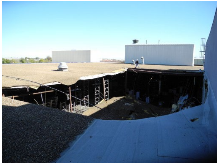
Figure 4. A view of the roof collapse. The new building addition is on the right.
