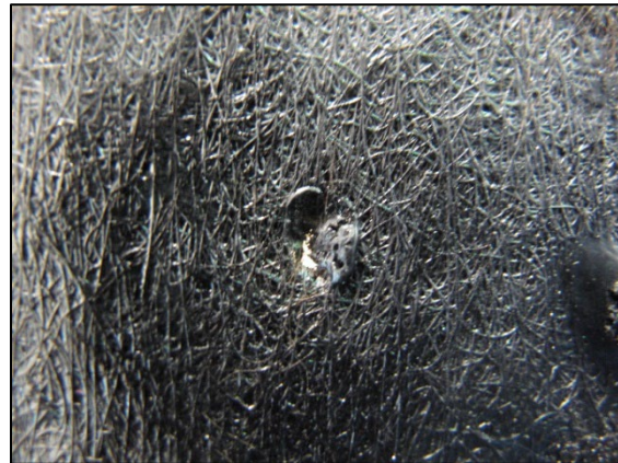
Figure 11: Adjacent felt ply indented and ruptured from the entrapped rock shown in Figure 10 (not consistent with impact)
