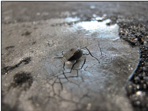
Figure 10: Small rock trapped between a sample's membrane plies, from an actual hail-damage investigation
