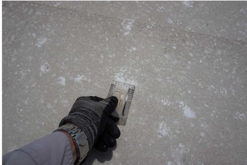
Figure 1. Burnish marks on a single-ply roof membrane.
