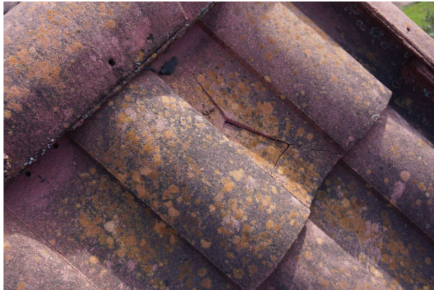
Figure 3. Fracture at a concrete roof tile. The fracture appears fresh and there is a large burnish mark coincident with the fracture location.
