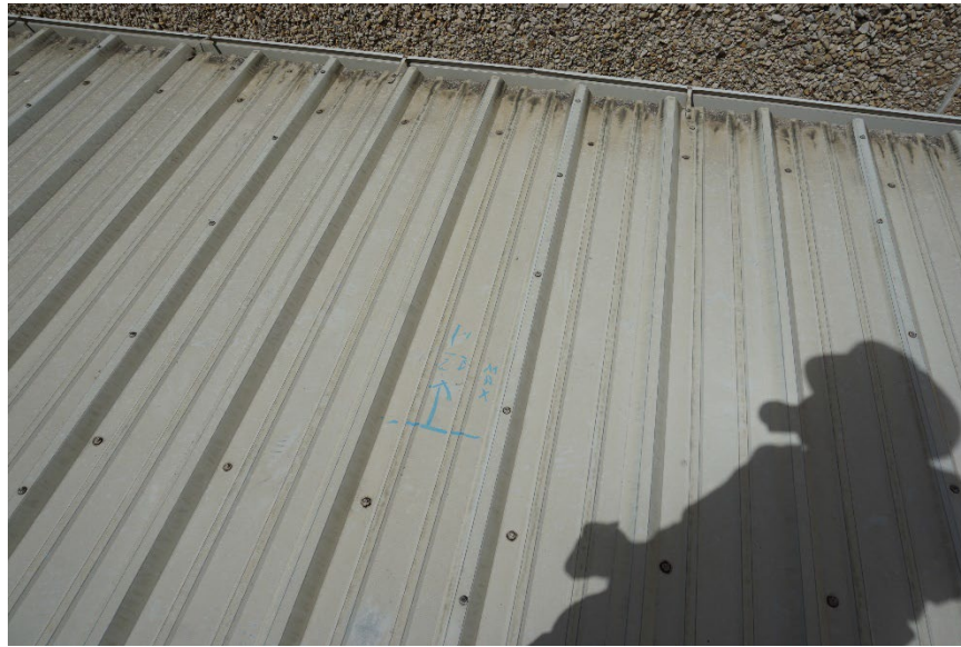
Figure 8. Lack of large burnish marks at the west portion of the low metal roof adjacent to the taller main building. The chalk mark denotes 1/2" [1.3cm] maximum burnish mark size at the area along the west side of the roof, close to the adjacent building.
