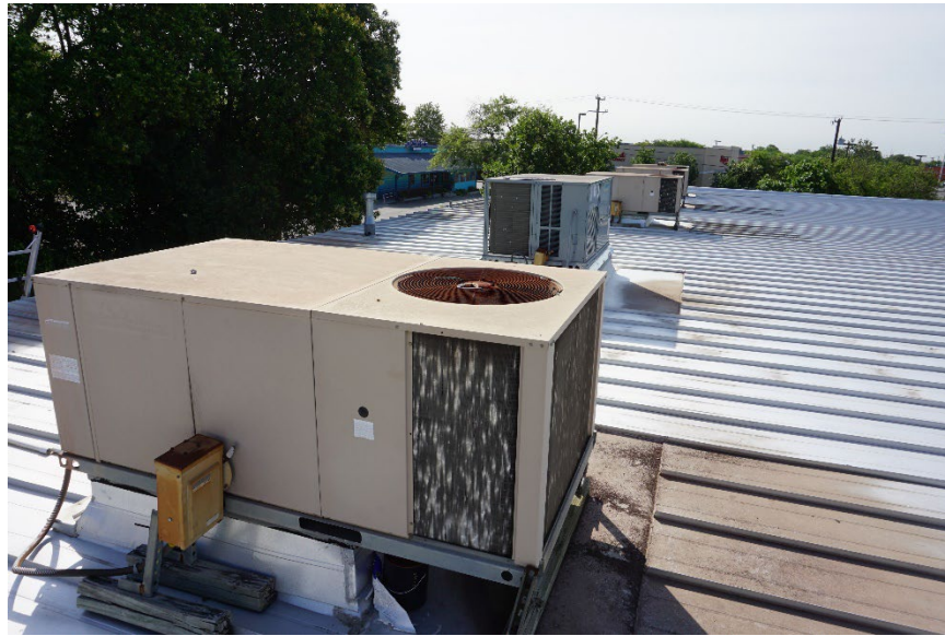
Figure 4. Older unit (foreground) with deformations throughout the coil fins, with a newer unit (in the background) lacking this pattern of deformation.
