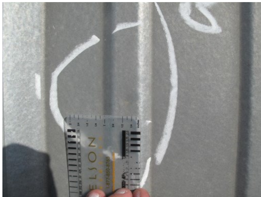
Figure 5. Circular indentation in metal panel roofing.
