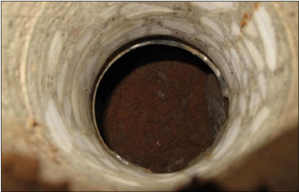
Figure 13: Representative view at Core 4 with a measurable void of approximately 6"
