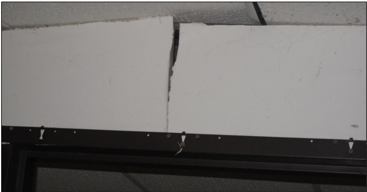
Figure 9: Wall and ceiling distress in close proximity to the fire riser
