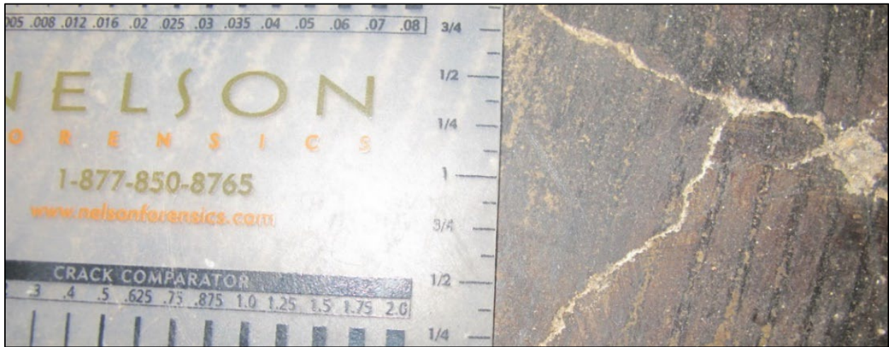
Figure 8: Concrete slab cracks with rounded/weathered edges
