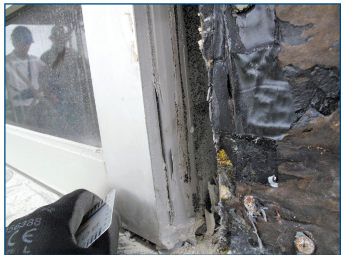
Figure 9 – Large gap at curtainwall jamb and no WRB or flashing wrapped in rough opening.
