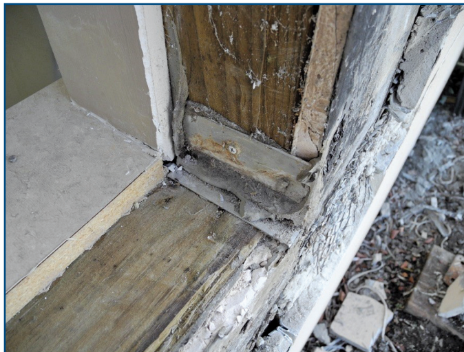
Figure 14 – End dams directly connected to rough opening rather than sill pan. Note the WRB terminating at vertical face of sheathing and not wrapped into rough opening.
