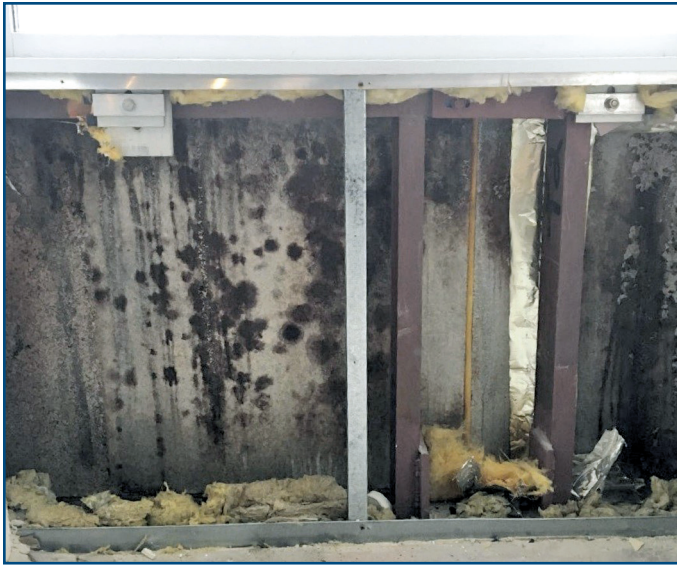
Figure 12 – Suspected fungal growth at back of granite panels. Exposed backer rod (yellow in color) for exterior sealant between granite joints (photo provided by client).
