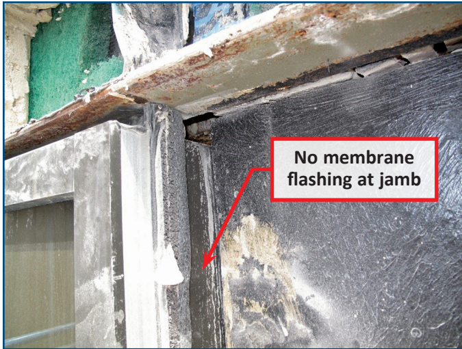
Figure 10 – No flashing integration of curtainwall jamb and WRB.
