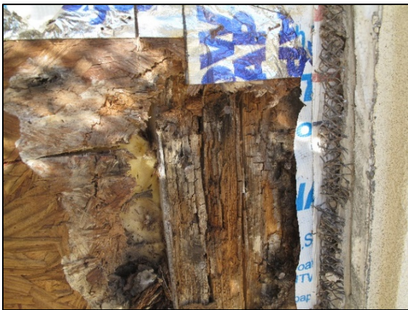
Figure 2: Deteriorated wood framing below a window
