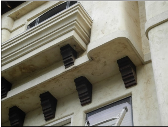
Figure 12: Soffit staining and lack of weeping provisions
