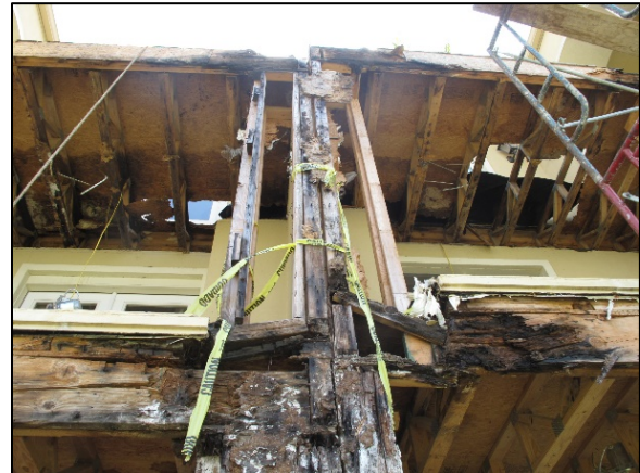
Figure 13: Balcony framing deterioration
