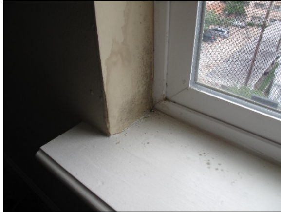
Figure 1: Moisture staining adjacent to window jamb
