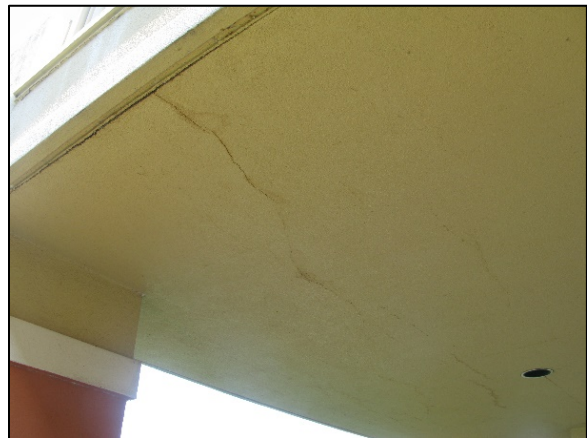
Figure 10: Fractured stucco at a balcony soffit
