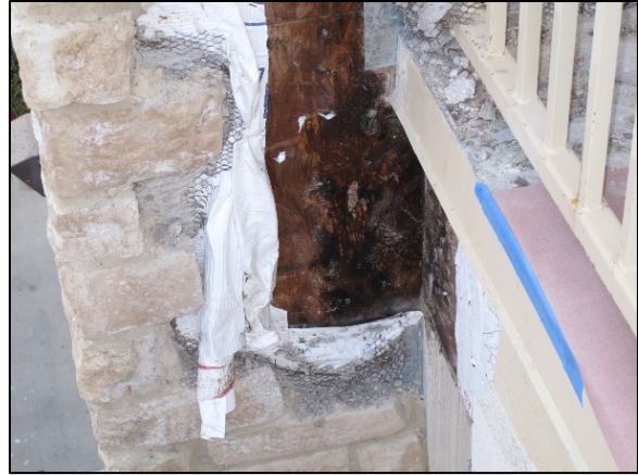
Figure 9: Deterioration of the sheathing at the balcony and wall interface
