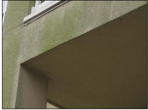
Figure 5: Lack of weeping provisions at soffit transition
