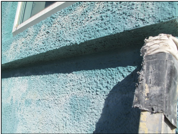
Figure 13: Staining at stucco below a window
