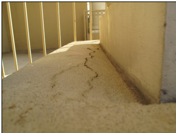
Figure 9: Fractured stucco at a column pedestal
