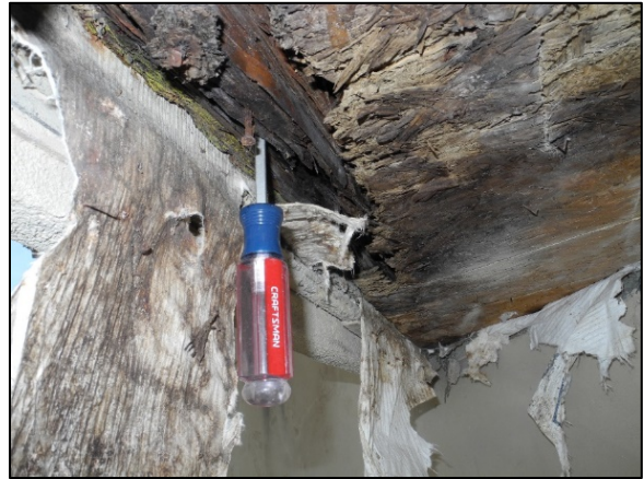
Figure 15: Structural framing deterioration at the soffit condition and one layer of building wrap
