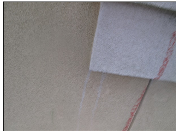
Figure 3: Moisture streaking below EIFS banding with no fracturing of the stucco
