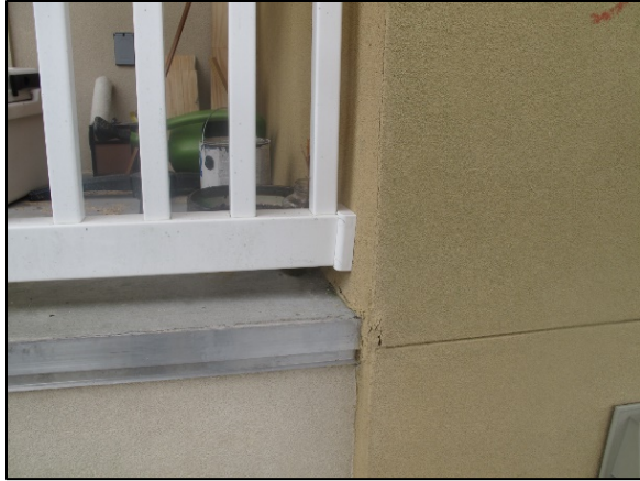
Figure 4: Stucco veneer in contact with concrete topping slab
