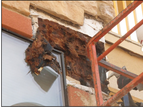
Figure 8: Deterioration of the sheathing at the head and jamb of a window
