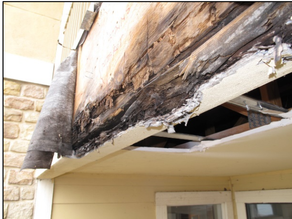
Figure 11: One layer of WRB at deteriorated framing conditions
