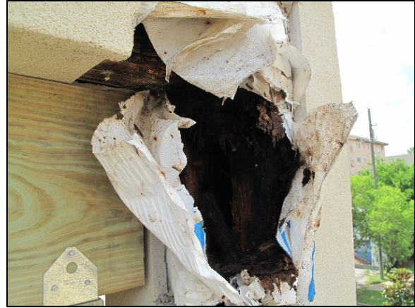
Figure 7: Deterioration of the structural wood framing at balcony column and temporary framing
