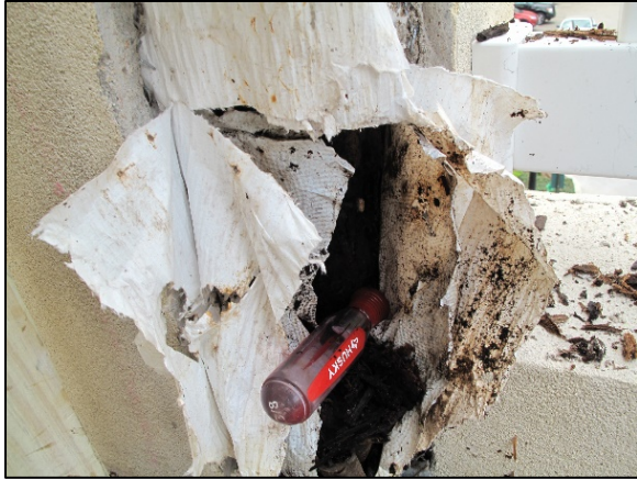
Figure 6: Deterioration of the structural wood framing at balcony column
