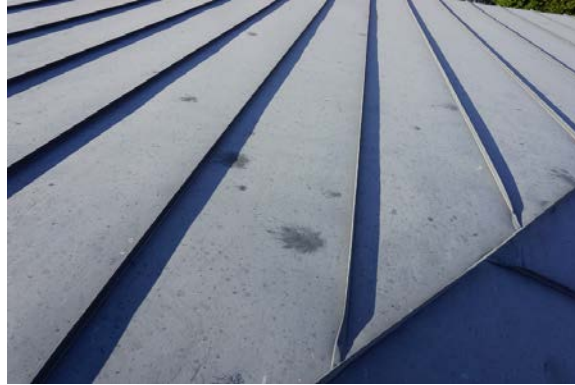
Figure 1. Burnish marks on metal roof panels with coincident indentations.
