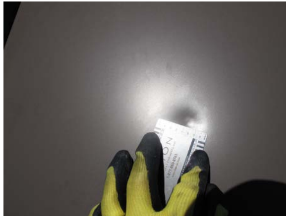
Figure 3. Indentation at metal roof panel.
