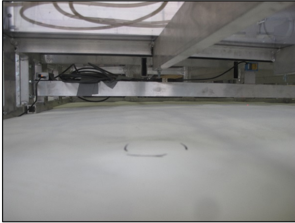
Figure 5: Membrane bubbling over insulation fastener locations at 105.0 psf
