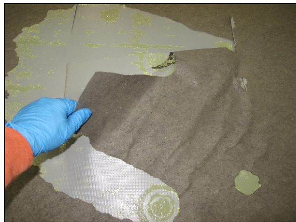
Figure 8: Underside of membrane at area where membrane separated from insulation
