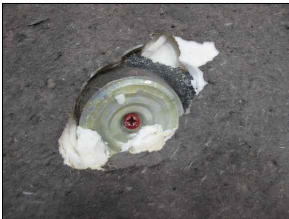
Figure 7: Polyiso insulation fractured at fastener
