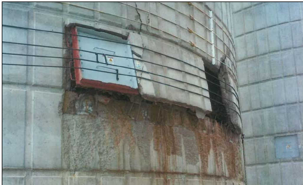
Figure 8. Additional view of silo wall failure at Jump 4
