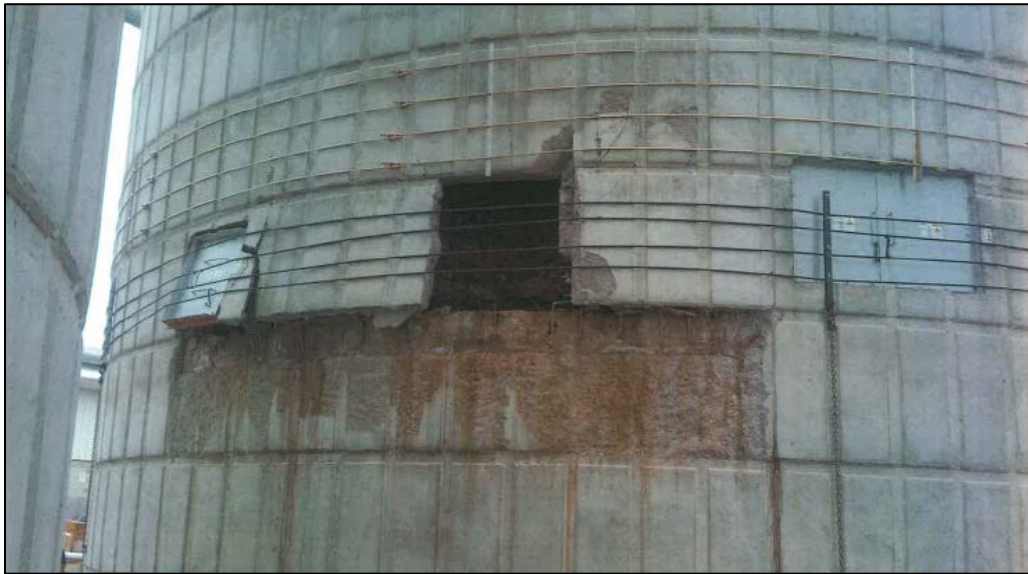
Figure 7. View of silo wall failure at Jump 4
