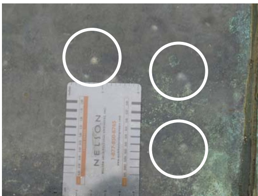
Figure 2. Hail Indentations to Copper Roof
