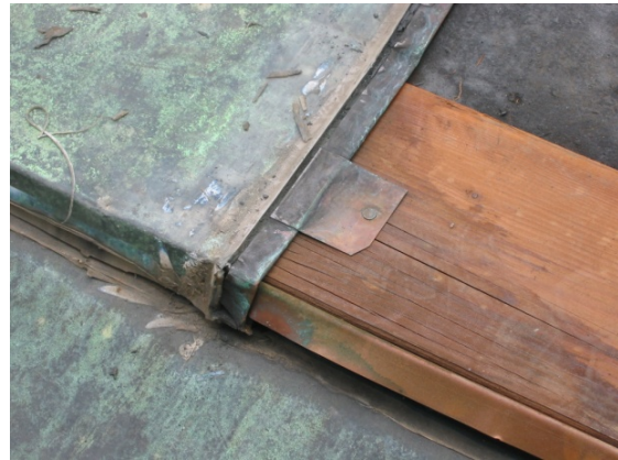
Figure 7. Copper Seam and Water Staining on Cedar Battens
