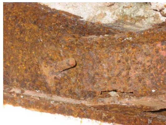
Figure 3. Corrosion of Steel Framing (Claimed as Hail Damage)
