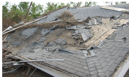
Figure 6. Typical roof distress
