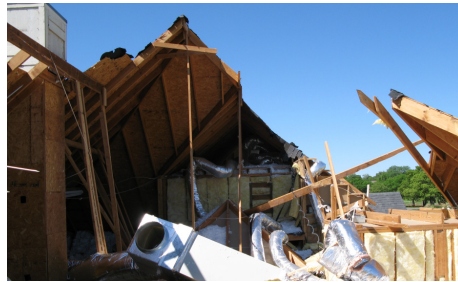
Figure 8. Roof framing distress
