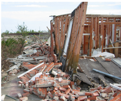
Figure 5. Brick veneer distress
