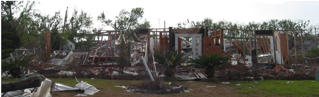
Figure 4. Typical condition of remaining structure
