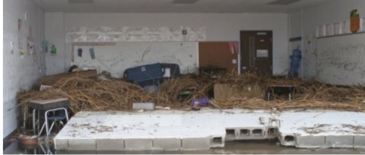
Figure 2. Collapsed CMU walls
