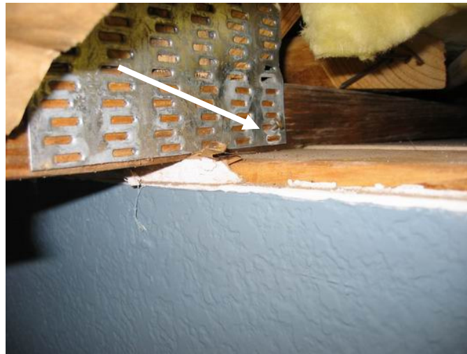
Figure 3. Truss bearing on a wall not designed as load-bearing. Note the nail connecting the truss to the wall (follow arrow).
