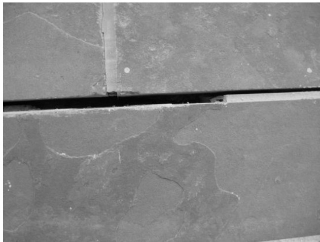
Figure 10. Veneer displacement and loose mortar above entry.
