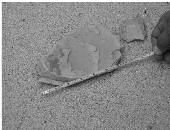
Figure 5. Piece of delaminated limestone measures 7" in length.
