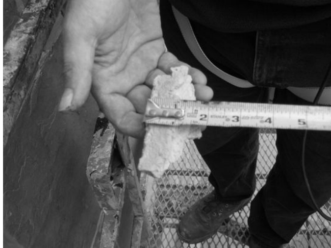
Figure 8. Depth only 1" at extracted mortar.
