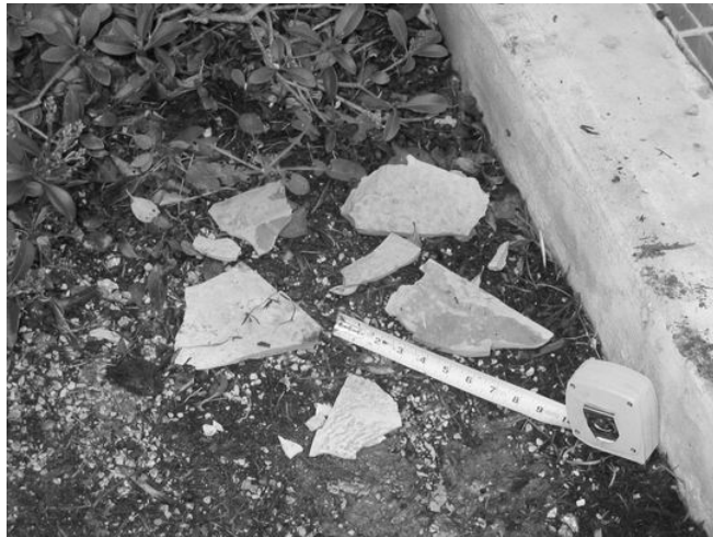
Figure 4. Pieces of delaminated limestone veneer on the ground.
