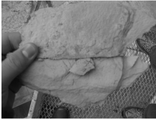
Figure 7. Delaminated stone pieces with no expansion joint.
