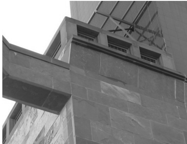
Figure 9. Angled stone veneer at fourth floor. There is no mechanical horizontal anchorage to the concrete structure.
