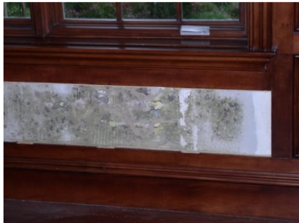
Figure 2. Mold on gypsum board behind removed wood paneling
