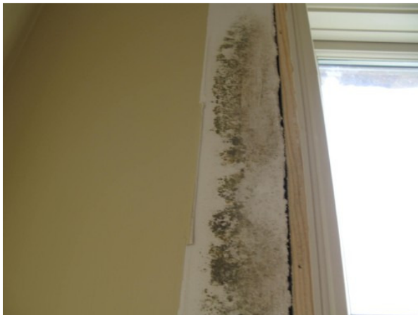
Figure 1. Mold behind removed wood trim
