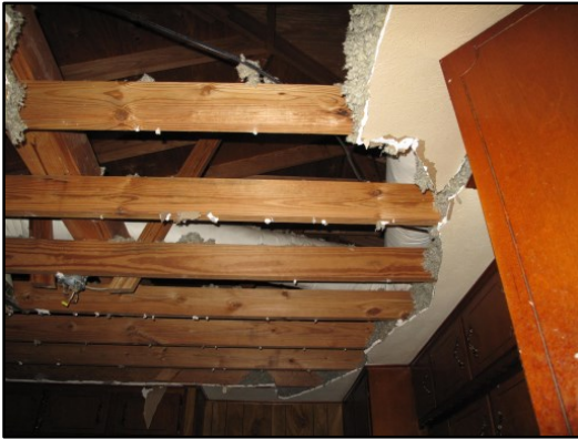
Figure 5. Collapsed Ceiling Finish
