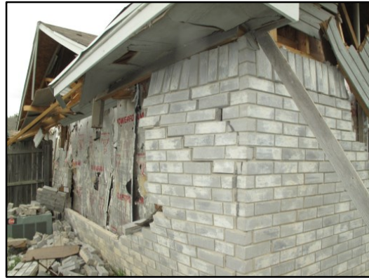
Figure 2. Buckled and Collapsed Veneer at Structure Exhibiting Severe Structural Damage
