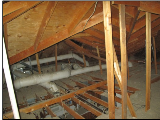
Figure 6. Collapsed Ceiling Finish
