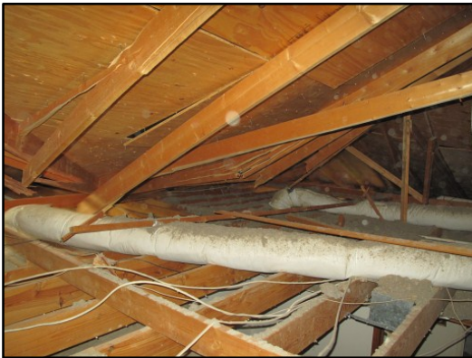
Figure 3. Fractured Roof Framing
