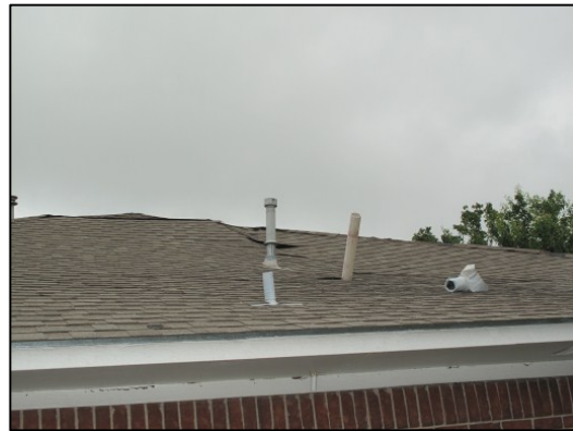
Figure 4. Shingle Distortion Isolated to Areas of Structural Roof Damage
