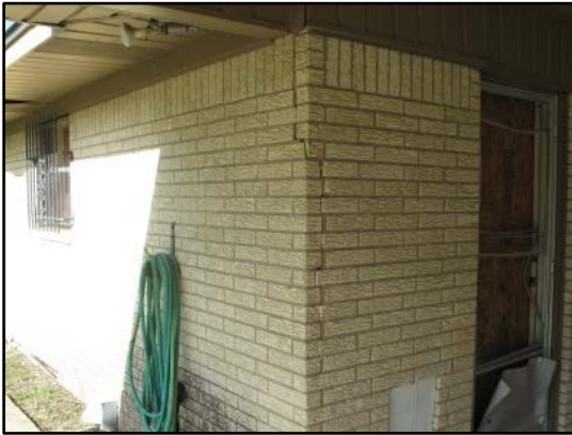
Figure 1. Near-Vertical Fractures at Exterior Corners
