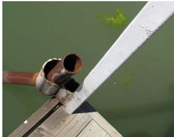
Figure 4. Failed anchor pole.
