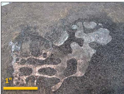
Figure 2 – Example of mopping void from a delaminated membrane sample
