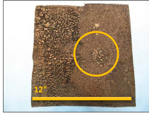
Figure 6 – Mopping voids below granule loss from Figure 5.
