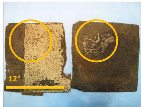
Figure 8 – Mopping void below flood coat loss from Figure 7.
