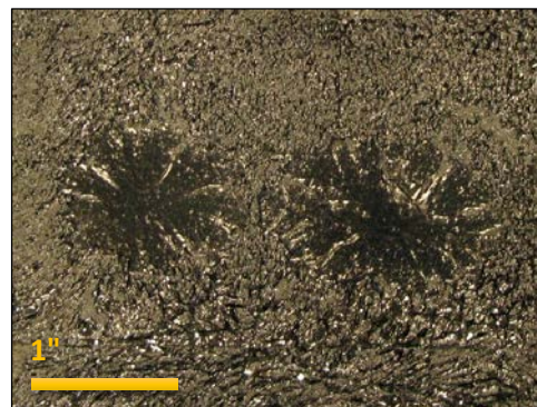
Figure 3 – Example of mopping voids from a delaminated membrane sample
