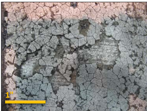
Figure 7 – Loss of flood coat over mopping voids in BUR membrane.
