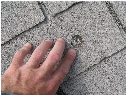
Figure 3. Hail impact mark on a roof shingle.
