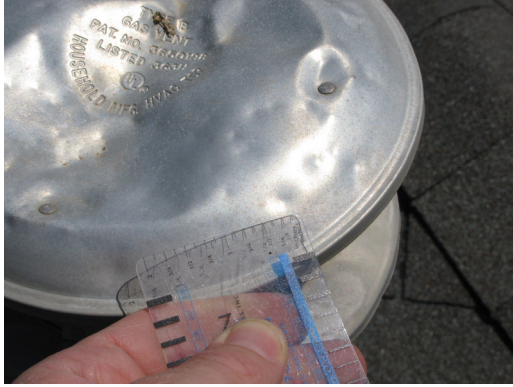
Figure 1. Hail indents on a roof vent cover.
