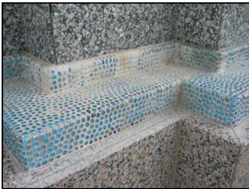
Figure 8. Moisture staining at base projection.
