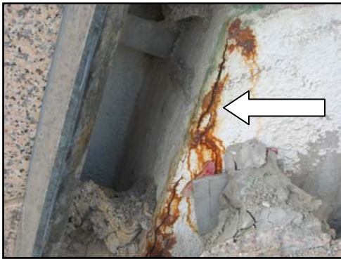
Figure 10. Corrosion at protruding corner of dome shell.
