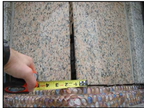
Figure 7. Separation at protruding corner near projection.
