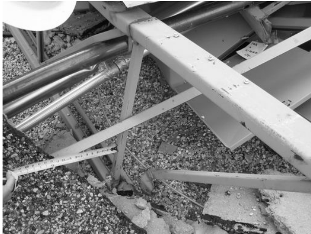
Figure 3. Typical joist geometry. Note the failure at the end web connection at the bottom chord.
