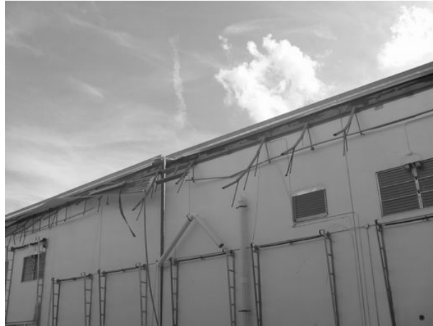
Figure 6. Failed joists. The webs failed at the bottom chord.
