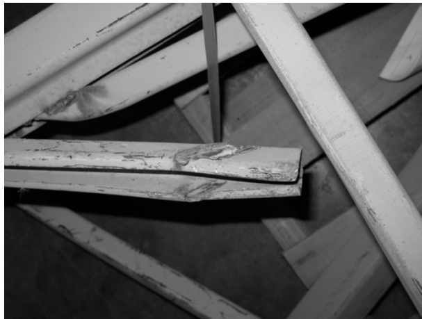
Figure 7. Failure at welded connection.
