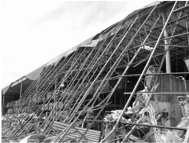
Figure 4. Collapsed joists. Note the lack of plastic deformation.
