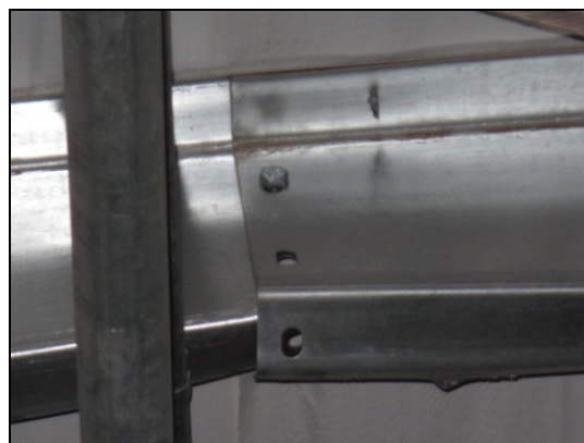
Figure 7: Missing bolt at splice
