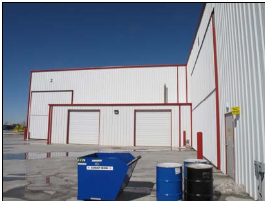
Figure 2: Southwest lower roof at internal corner of upper roof structure
