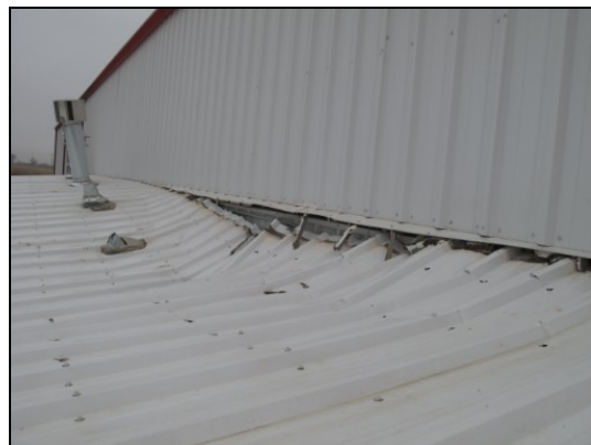
Figure 5: Roof deck pulled away from upper roof structure
