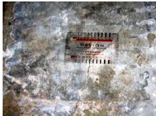
Figure 8: Shrinkage fracture at concrete substrate.
