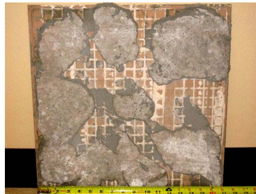
Figure 10: Poor mortar coverage at underside of tile.
