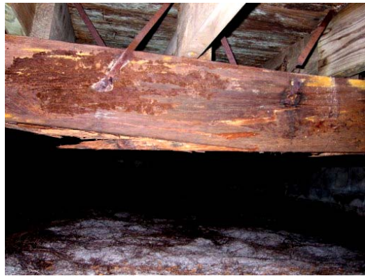
Figure 6: Deterioration of wood framing below tile floor system.
