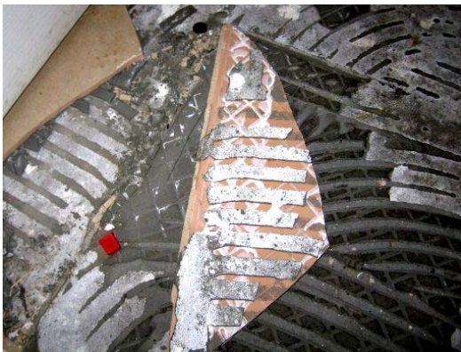
Figure 9: Deleterious material at mortar and substrate below.
