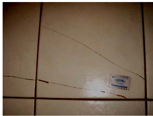
Figure 4: Fractures at tile from rolling load.
