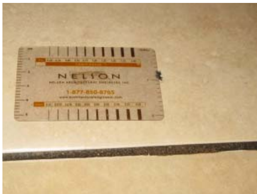
Figure 3: Impact fracture at tile.
