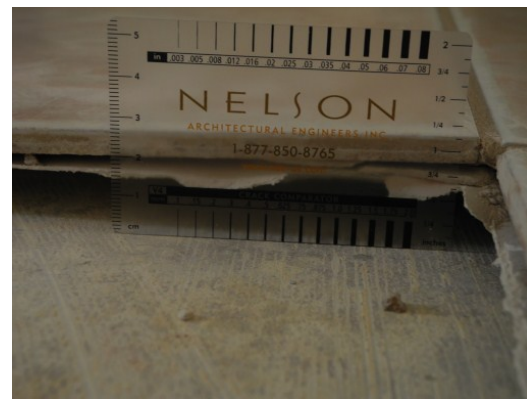
Figure 2: Void created by tile buckling.
