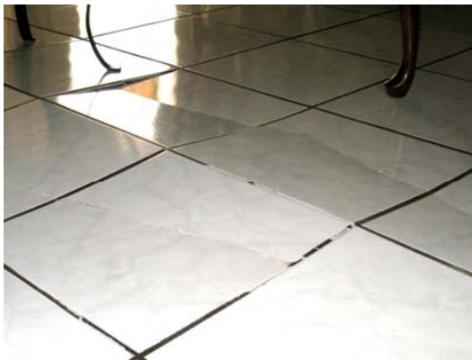
Figure 1: Buckling of tile flooring on slab.
