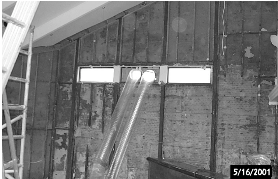
Figure 2. Water and termite damage at interior wall.
