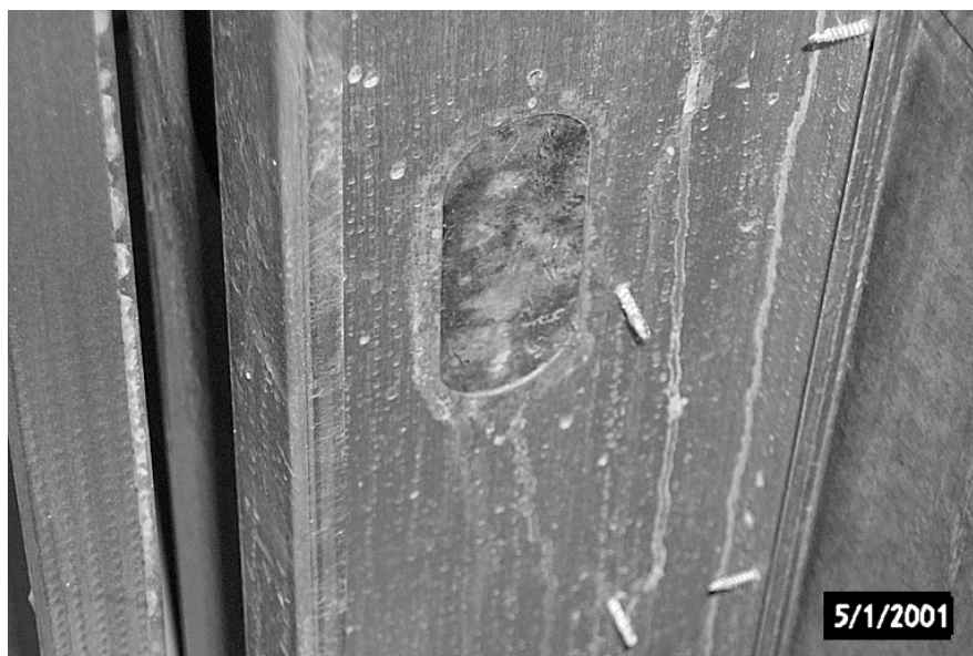
Figure 7. Streaking at metal studs and fungal growth at sheathing.
