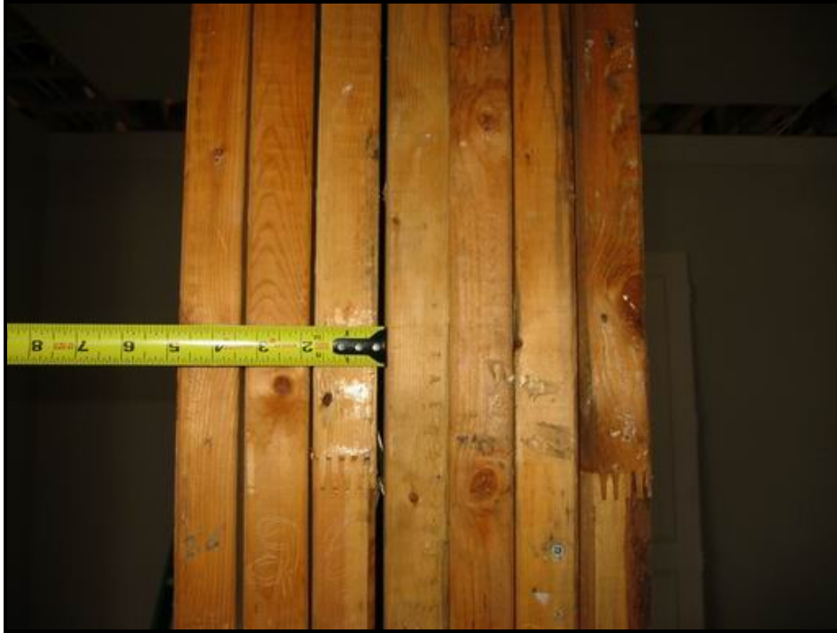
Figure 3. Measurement at mid-height of columns is 3/16". The studs have displaced laterally and are also separated individually.
