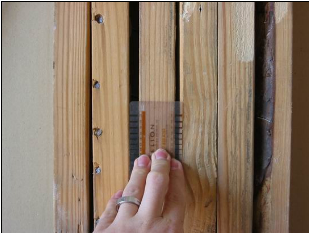
Figure 6. Nails attached near the edge of a stud in a "stud pack".
