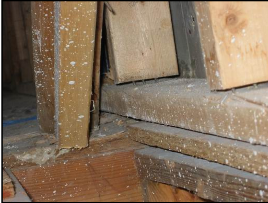
Figure 5. Separation of framing at attic level above a heavily-loaded column.
