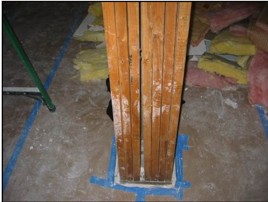
Figure 2. Bottom of two adjacent stud groups. The left group exhibits perceptible bowing. Measurement between columns was 1 1/16" at the bottom.
