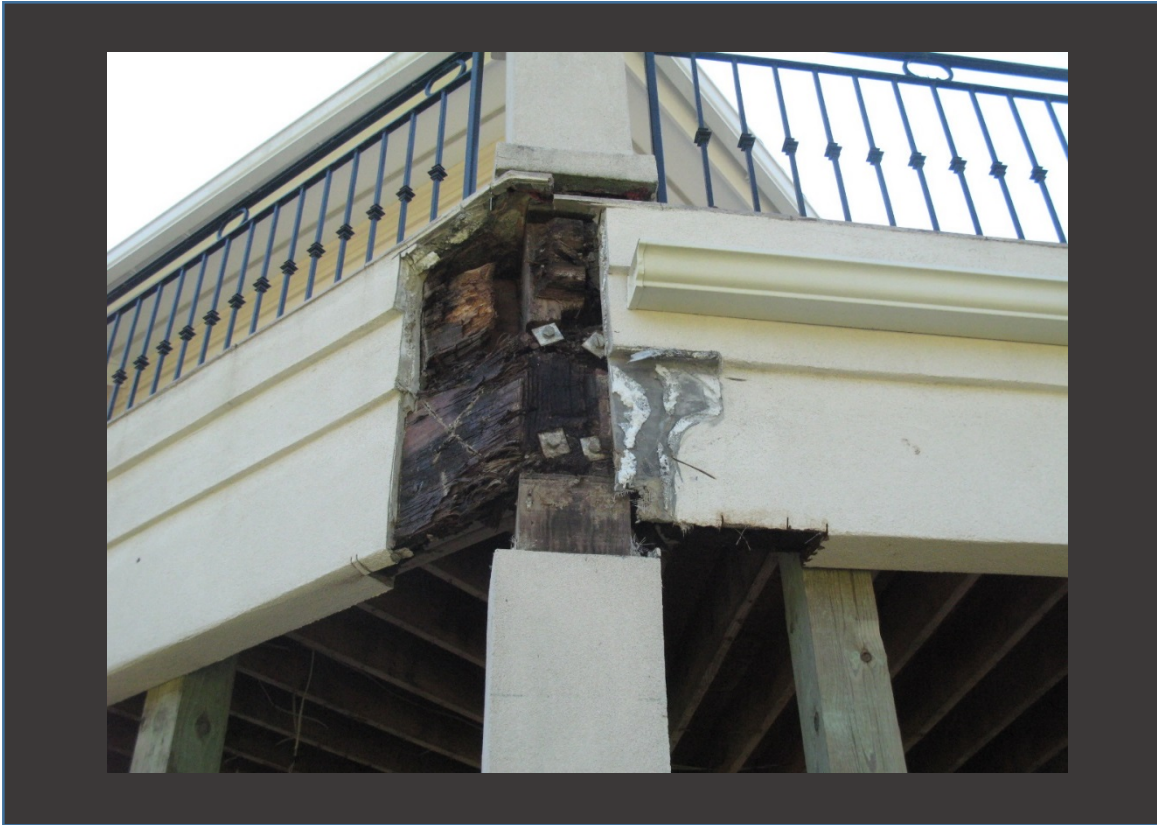
Figure 1: Exposed balcony assembly
