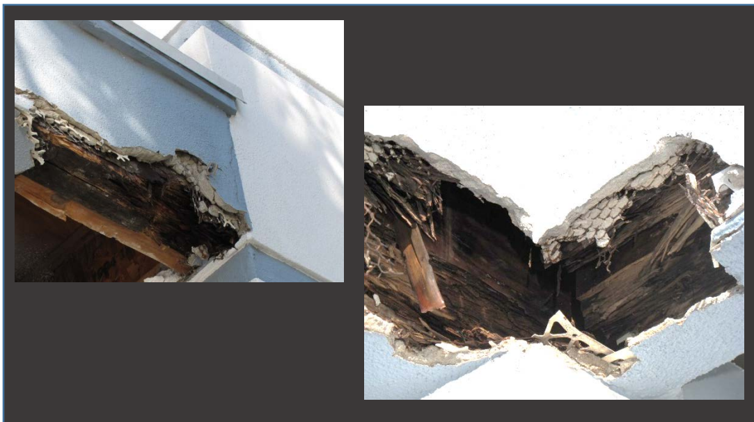
Figure 6: Deterioration of LVL beams
