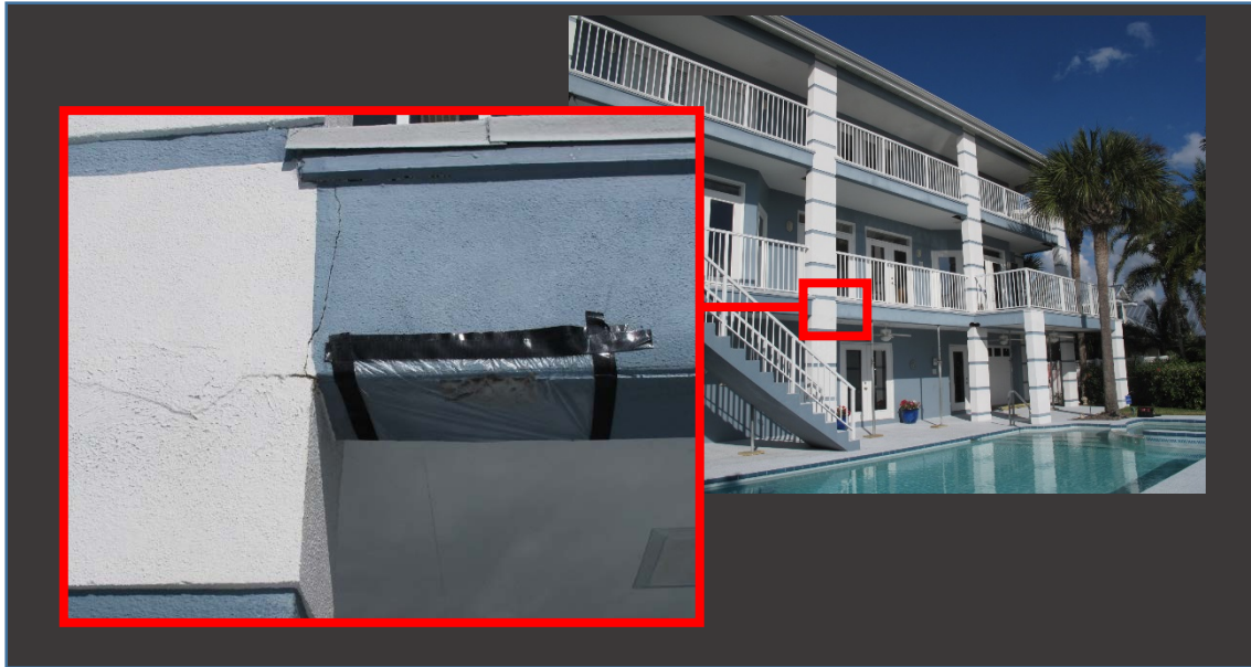
Figure 5: Stucco veneer distress at balcony beam and column interface
