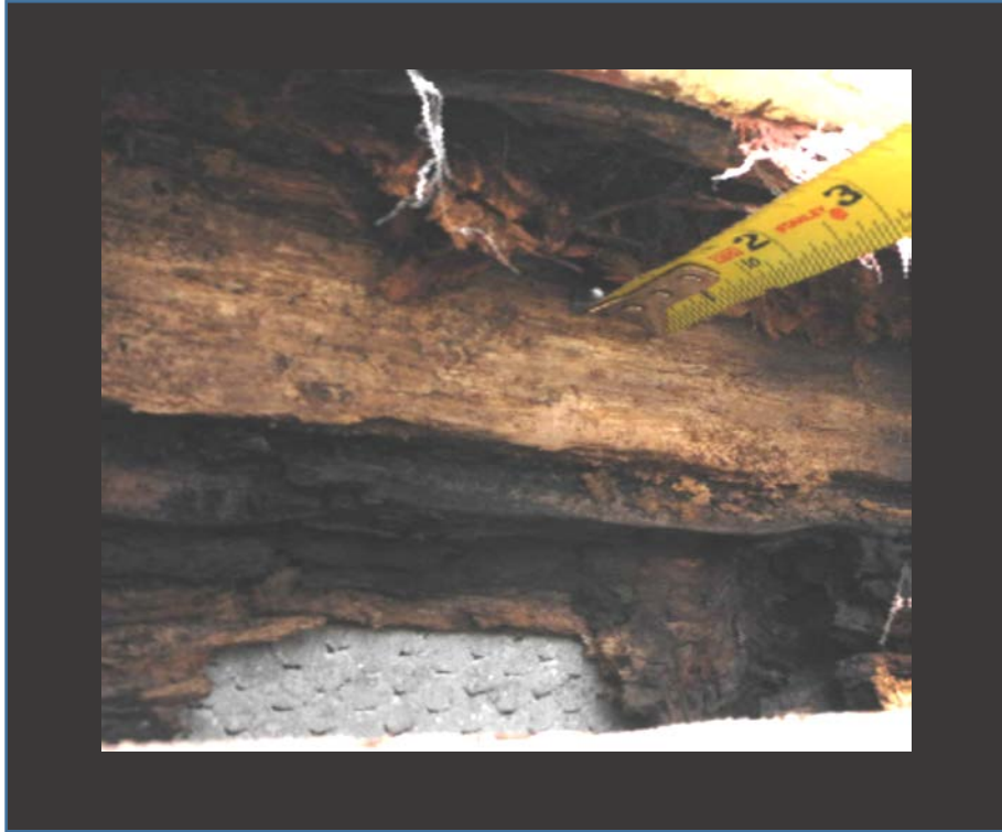
Figure 4: Deteriorated beam with exposed interior face of veneer
