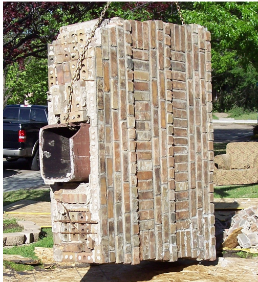
Figure 2. Solid Masonry Core Formerly at Top of Chimney
