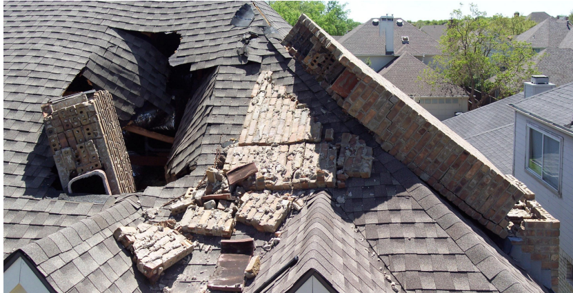
Figure 3. Collapsed Section of Chimney Above Children's Bedroom
