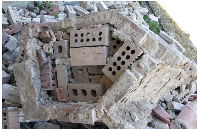
Figure 7. Lack of Mortar and Interlock at Masonry Core
