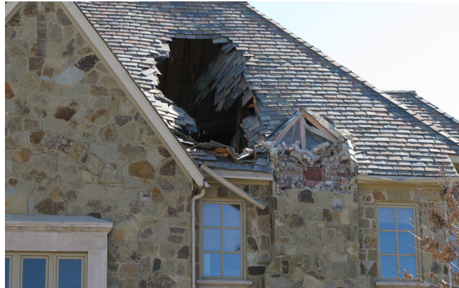
Figure 6. View of Collapsed Chimney
