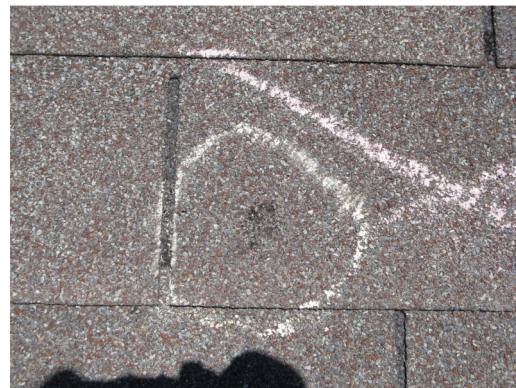
Figure 4. Hail impact mark on a roof shingle.
